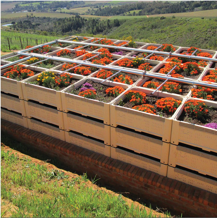
Uva Mira Mountain Vineyards, Stellenbosch Domestic sewage and wine cellar effluent treatment Treated water used for irrigation
