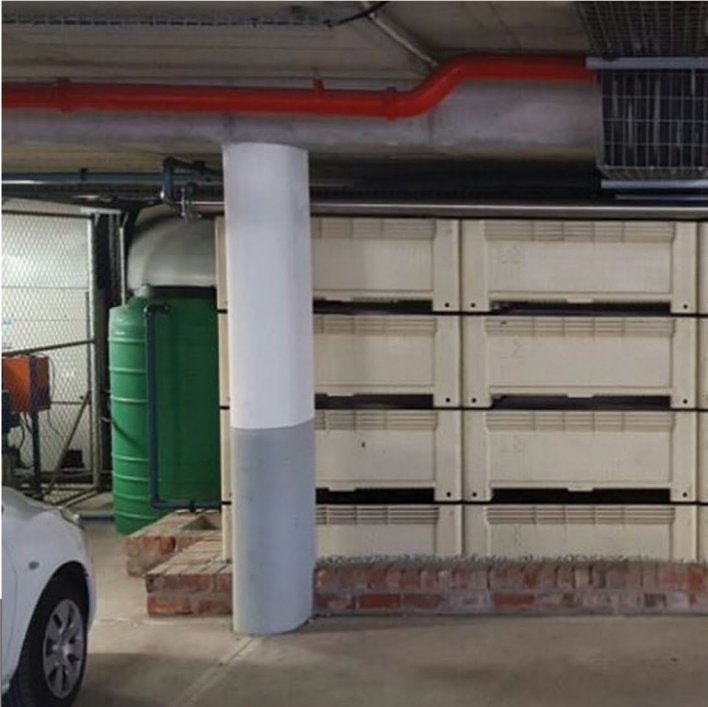
Old Mutual, The Estuaries, Century City, Cape Town Office block waste water recycled via The SOG Trickling Filter™. Additional RO reverse osmosis ensures potable water quality.
